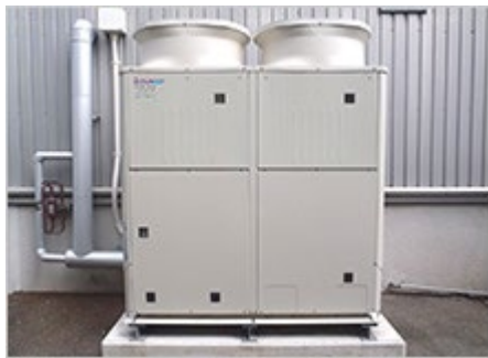
Chiller equipment upgrades at the Fukuoka Plant (Energy saving)
